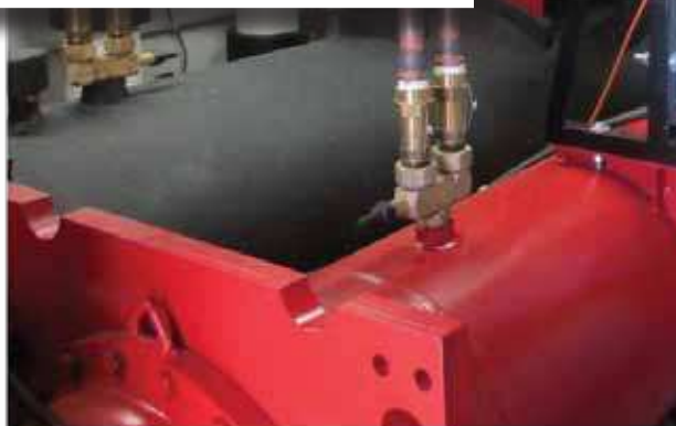
The MagLev compressors are controlled by Multistack’s FlexSys controller.
