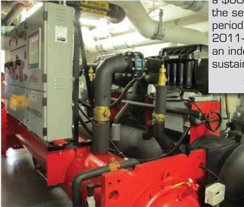
The 300-ton Multistack chiller at Windy Hill Hospital uses MagLev™ compressors for optimum efficiency and reliability while virtually eliminating compressor maintenance needs.
