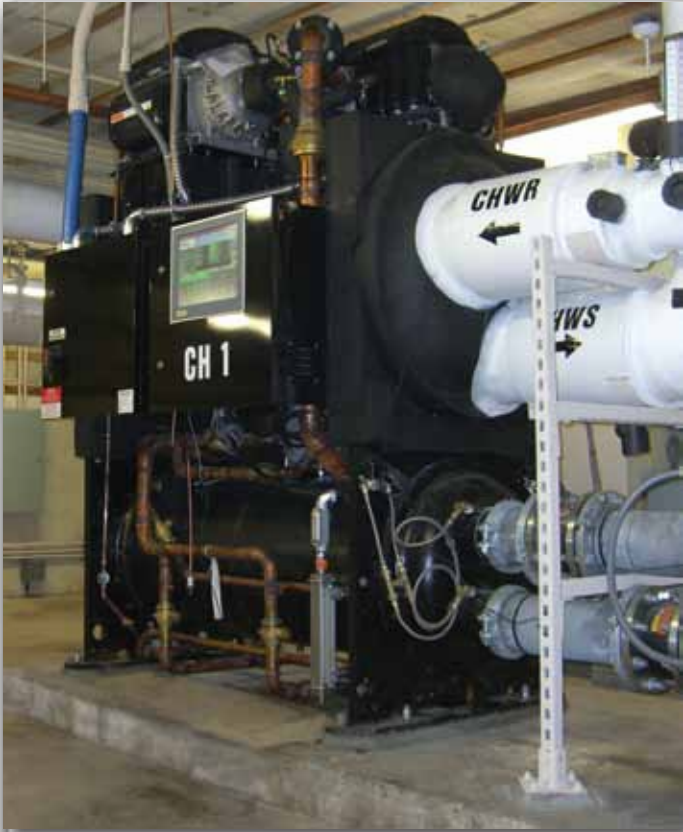
Moore Hall is equipped with two 160-ton Multistack chillers with the MagLev™ bearing system for high efficiency, high reliability and low maintenance.
