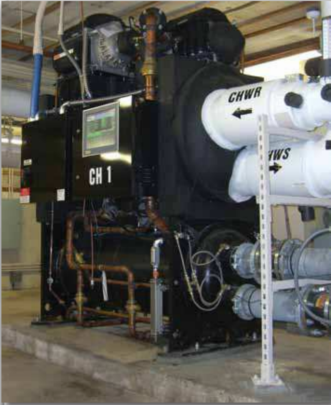
Moore Hall is equipped with two 160-ton Multistack chillers with the MagLev™ bearing system for high efficiency, high reliability and low maintenance.
