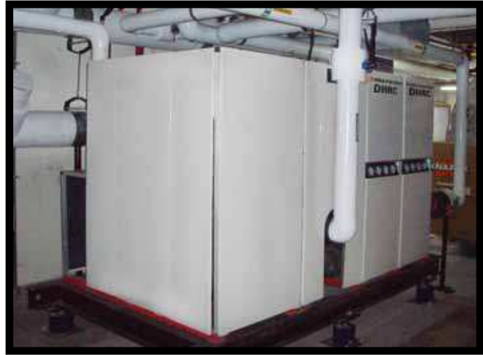
Inside the equipment room of the Embassy, sits the Multistack DHRC
