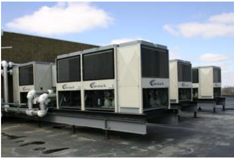
Four banks of Airstack chillers provide 330 tons of cooling for Central Blood Bank.
