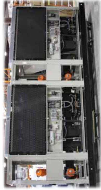
Refrigerant specialties and heat exchangers easily accessible on air- and water-cooled arrays. DDC controller on each module displays refrigerant temperature and pressures.
