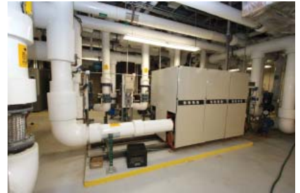
The Geo-H/C at KVHS has three 50-ton modules, with the piping and base sized for the addition of two more modules.
